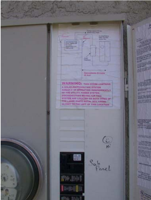
Figure 13 Sign at service entrance required by 702.8
