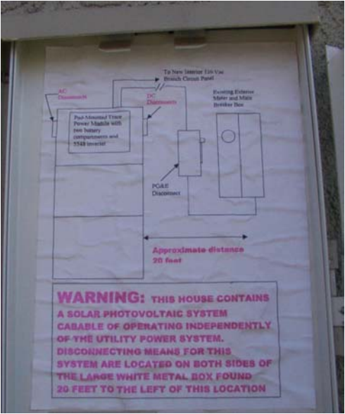
Figure 14 Close-up of sign for emergency personnel
