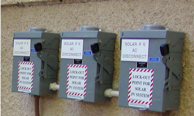
Figure 12 PV System Disconnect Signs
