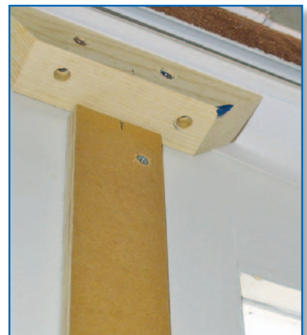
Inside view of the top of a door pair with stop block. A trim strip and weather stripping reduce air infiltration.
