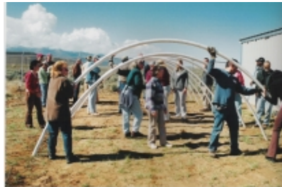
Figure 2. Bending the 2-in. x 20-ft. PVC pipe and setting them on 1/2-in. rebar stakes.
