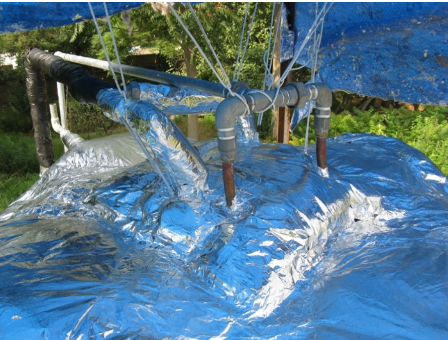
The tank was wrapped in a couple of layers of glass wool insulation.
