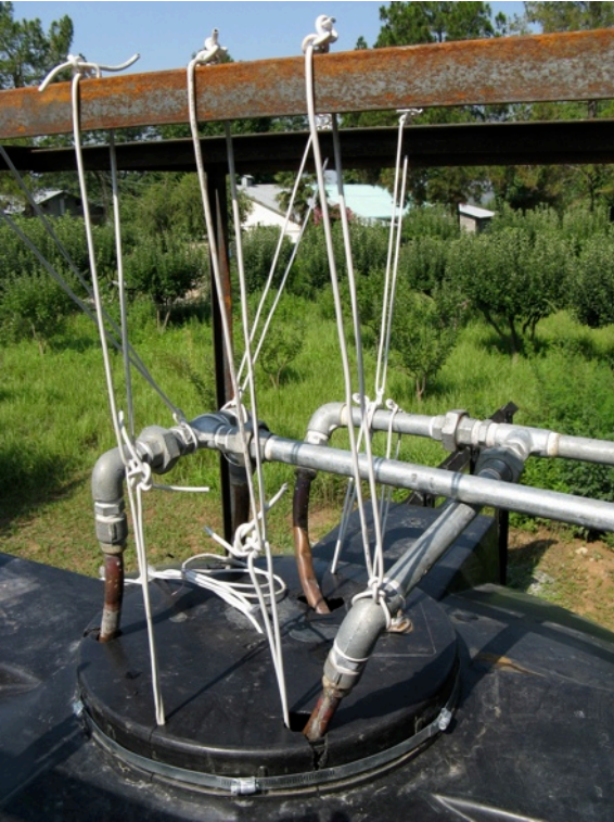
Copper coils suspended near the top of the tank.
