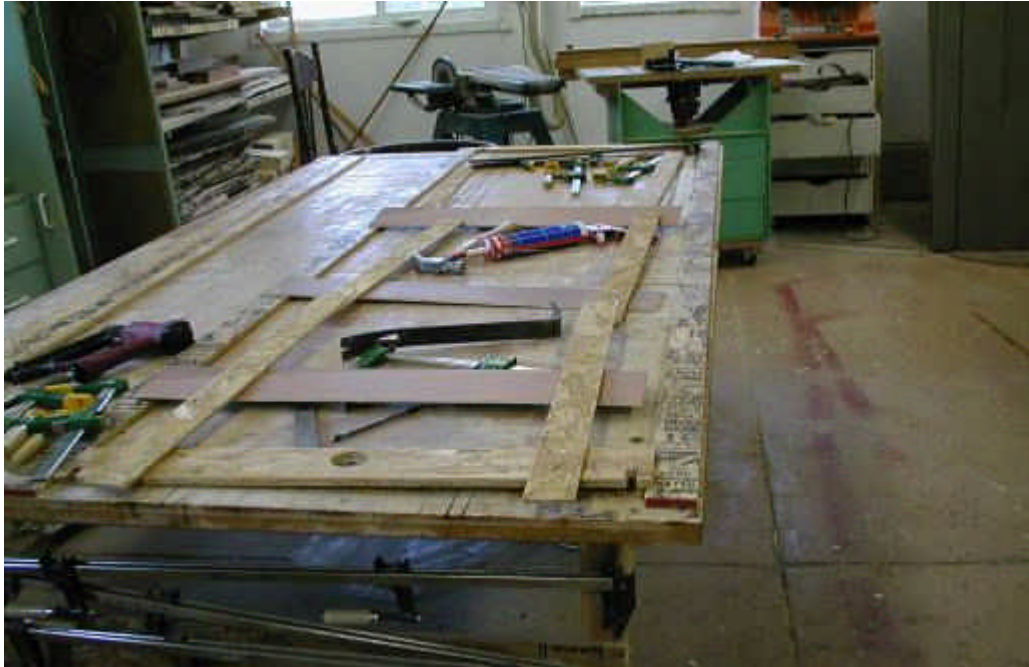
Pieces of framing laid out for assembly. A pneumatic brad nailer and construction adhesive is all that is used. A square table is nice to get the frame assembled square.
