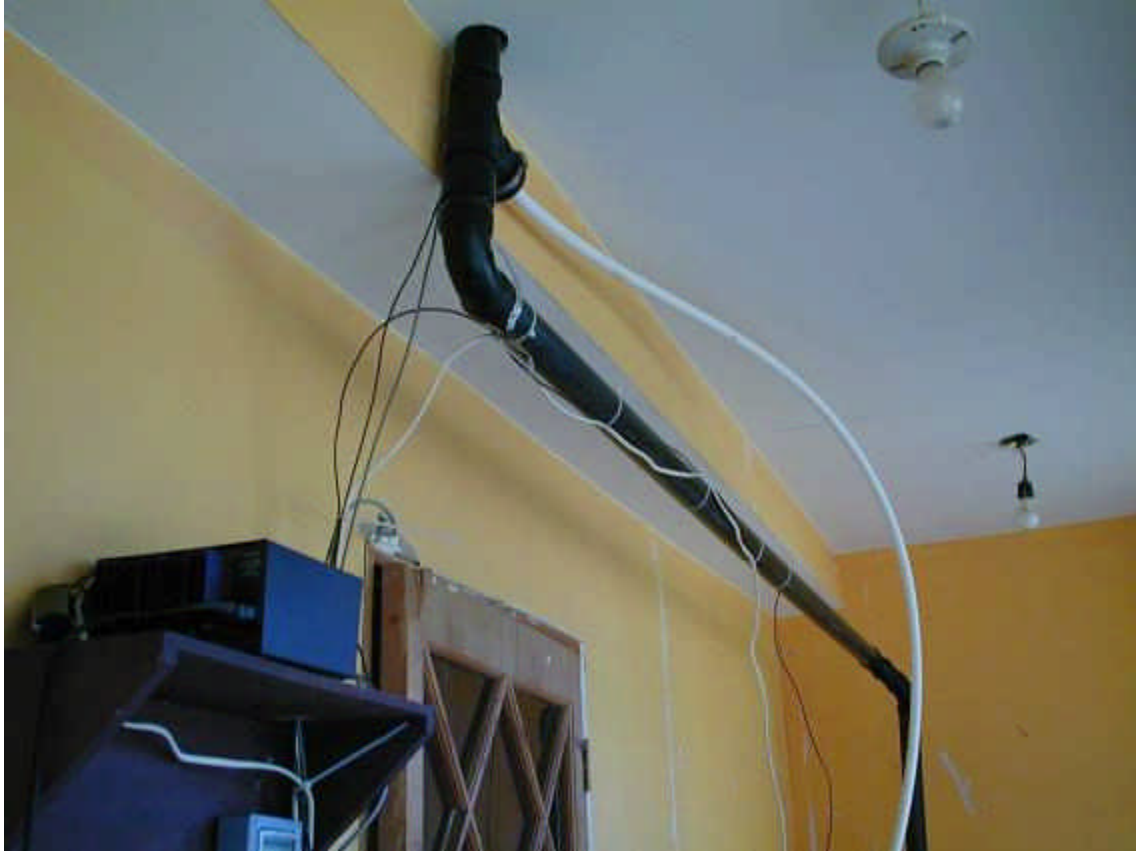
The feed and drain lines feed down thru the roof from the collector. The feed line enters thru a sanitary tee and a rubber test cap.
