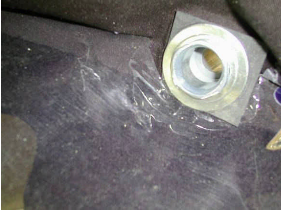
A view from the inside of the funnel. The chase nipple a reducing washer and an EPDM rubber washer installed.
