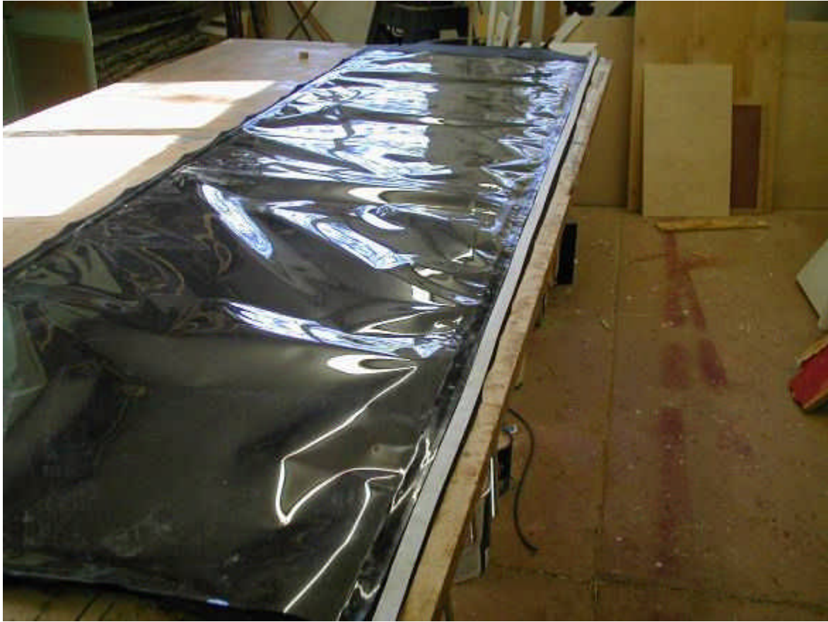
Fabric adhesive applied, paper backing still on. This forms the second seal of the standing seam edge.
