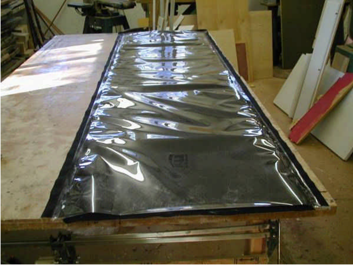
The side seams finished with the first half of the standing seam.
