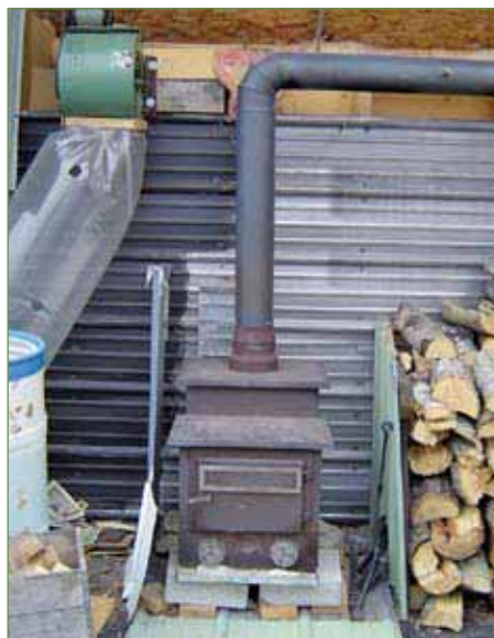
A wood stove supplements heat in cold weather. Heat from the stove is circulated to the greenhouse by a furnace fan that blows the hot air through a poly duct.
