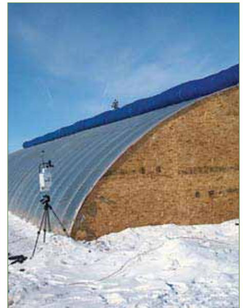
Partially unrolled thermal blanket on the greenhouse at Elie. A problem developed with the blanket when a tear in the plastic outer layer allowed rainwater to soak the insulation. In February, the blanket froze in place after it was unrolled, making it difficult to roll up and down.
