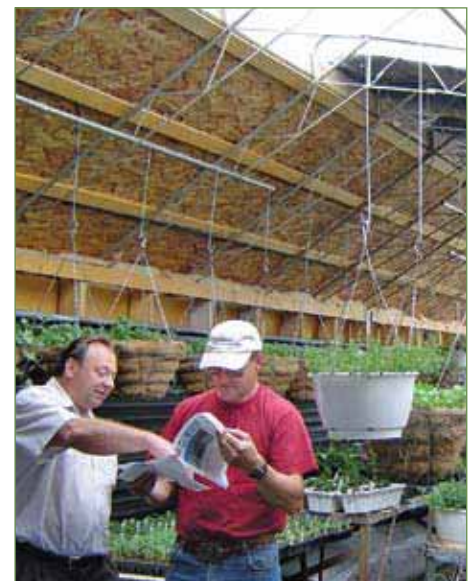
The steel ribs, the sand-filled rear wall, and sloping section of wall shown here are all standard features of the solar greenhouse at Ashern. Steel ribs are handy for hanging plants. The sloping section of wall will be clad in white or silver roofing tin to reflect sunlight onto the plants.
