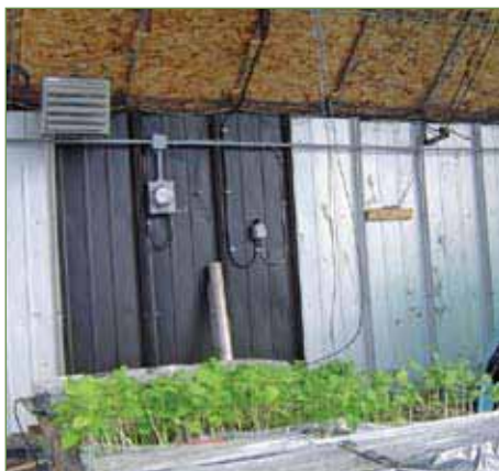
Second chamber in the greenhouse at Elie, February 7, 2006. One of two 5-kW GX agricultural electric unit heaters, top left, helped keep plants warm. Note section of rear wall, painted flat black to absorb solar heat.
