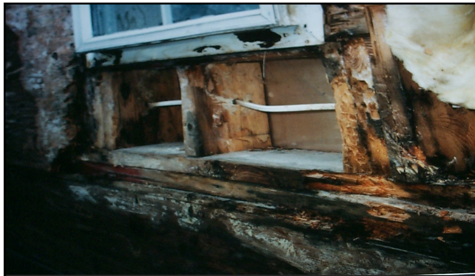
Figure 1 Damage due to moisture inside a wall.
