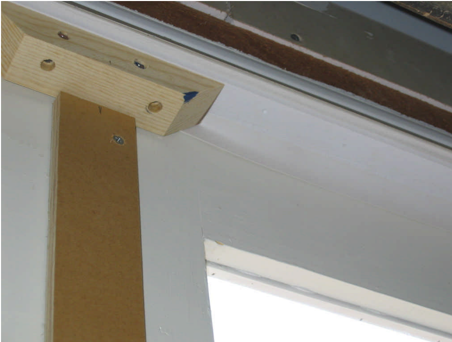
Door stop and sealing strip where doors meet. The white Vinyl weather stripping is just visible along the top of door. One of the Acrylic panels is visible in loser right.
