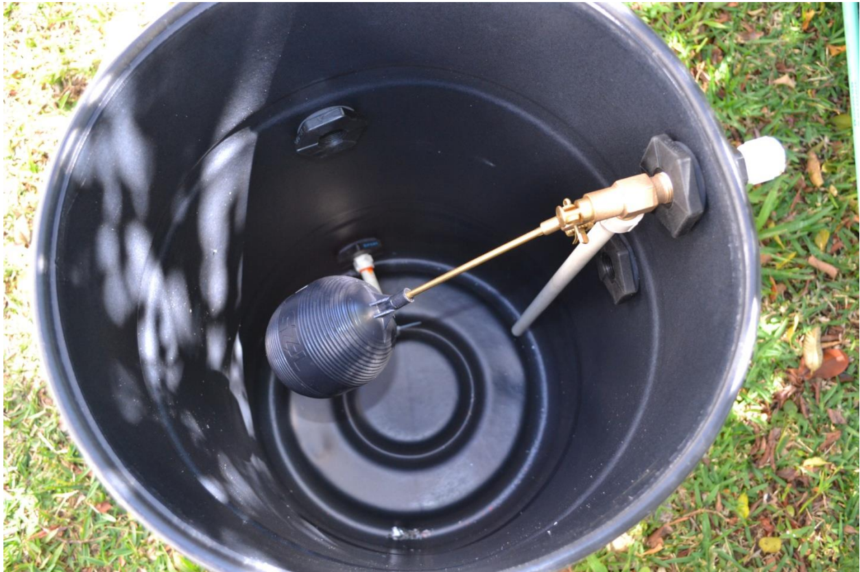
The intake valve with line feeding water to bottom of tank
