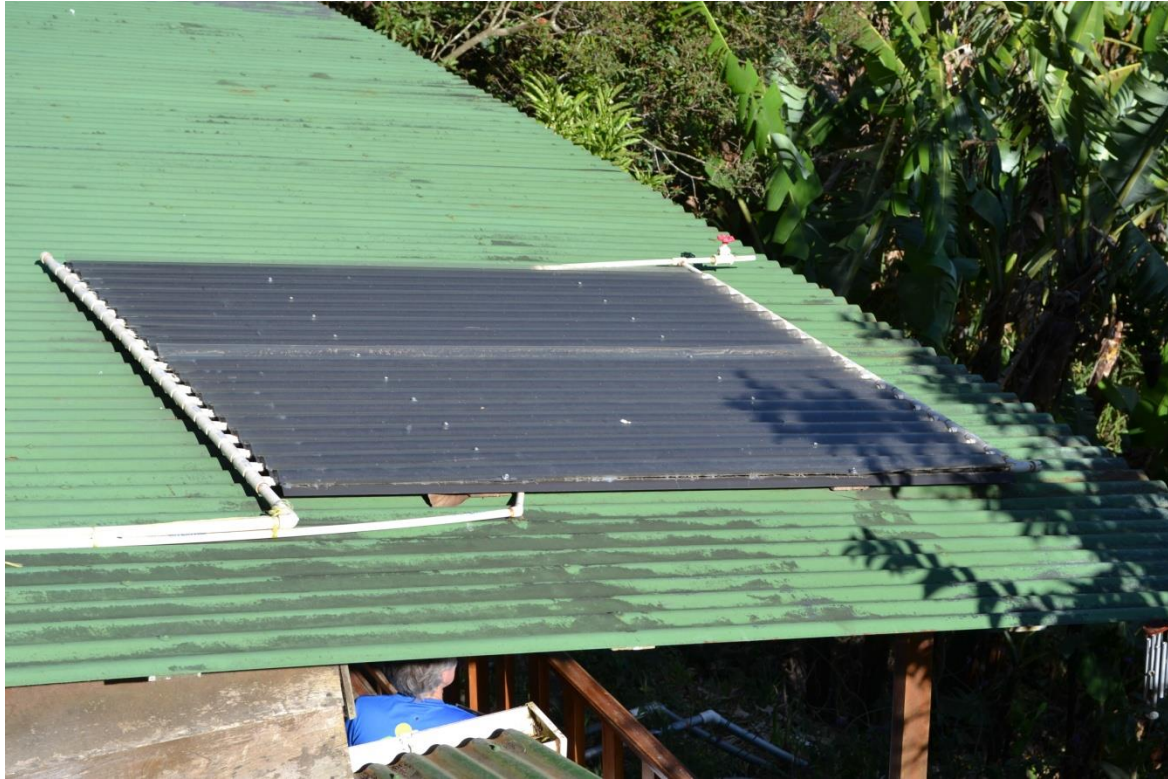
Installed and ready to make hot water
