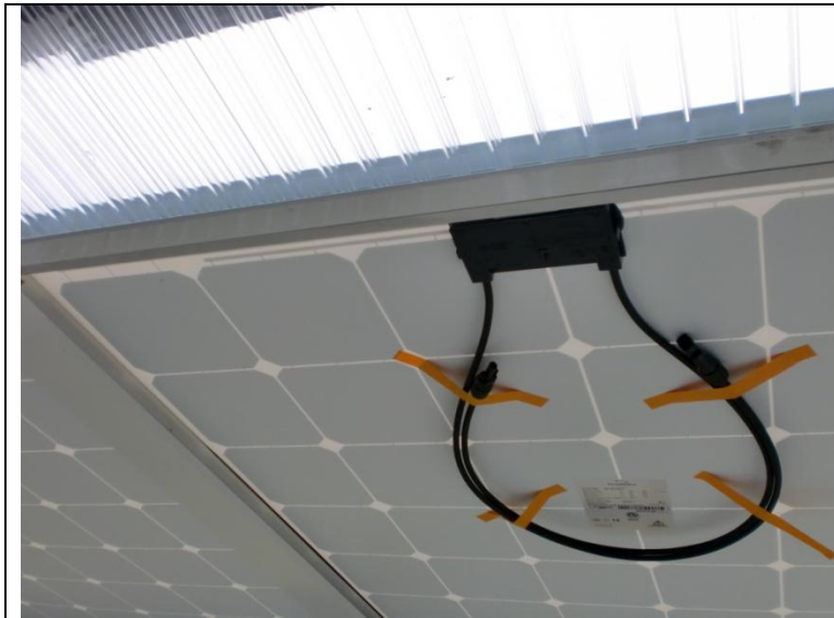
Underside of Solar World SunModule 255 Mono panels, showing “white space” around PV cells within the panels. The PV-module electrical cables seen here were not yet connected at the time of the photo.
