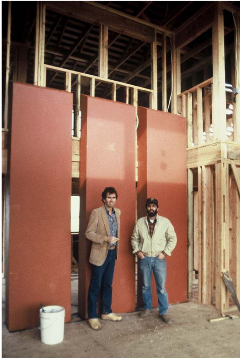
Denny Long with triple tank installation
