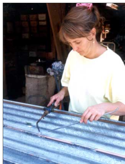
Robyn carefully applying heat and home-made solder in order to join the copper riser tubing to the galvanised corrugated iron.
