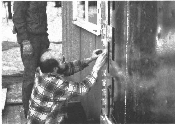
Laying out the EPDM End Closure Strips with a Scrap of Industrial Siding
