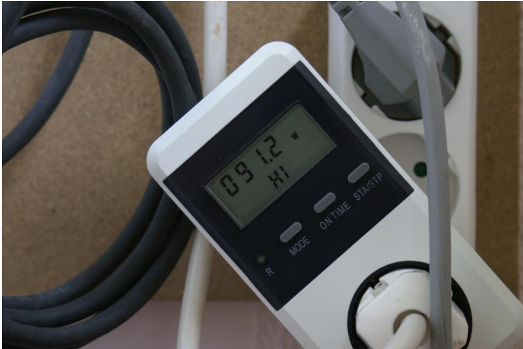
The ELRO M12 production meter with 91W of home build solar power.
