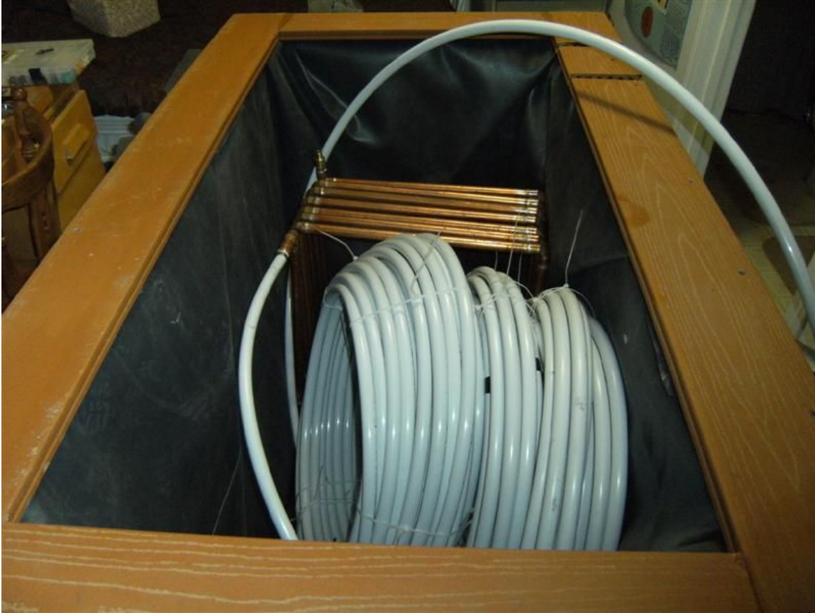
Partially connected PEX and copper combination heat exchanger
