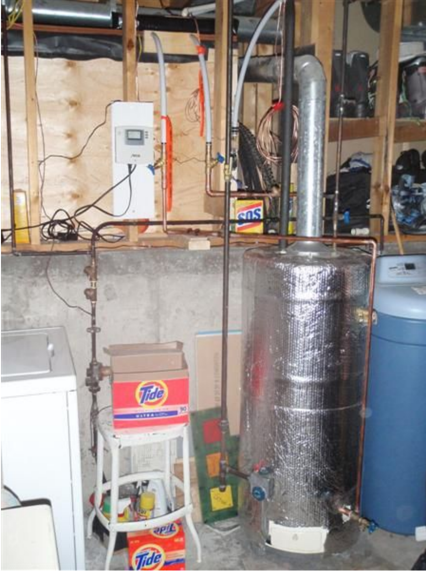
Setup with tank in background, controller, plumbing, and hot water tank
