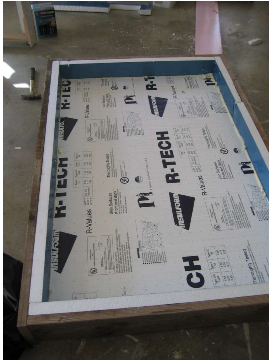
The basic box before the poly liner was put in. The insulation panel sits right on the ground.
