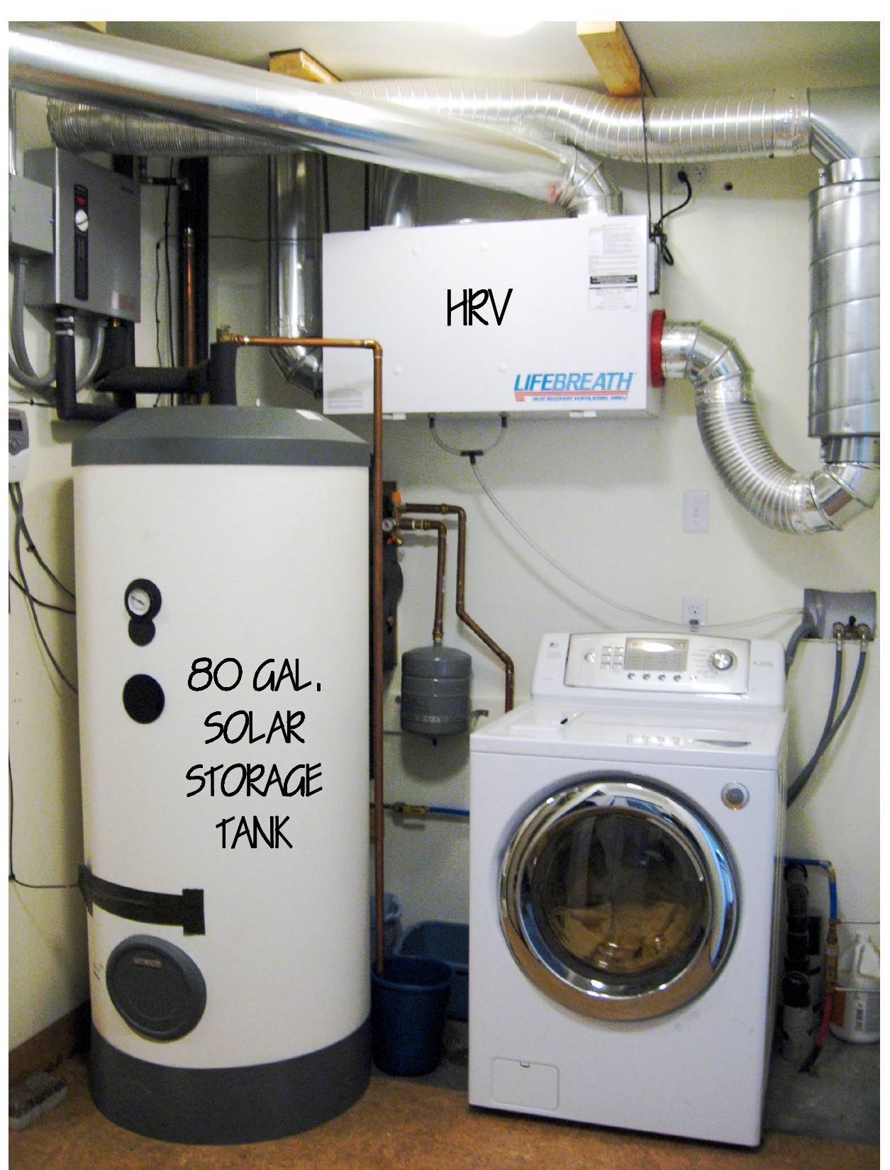
COMPACT CENTRALIZED UTILITY ROOM
