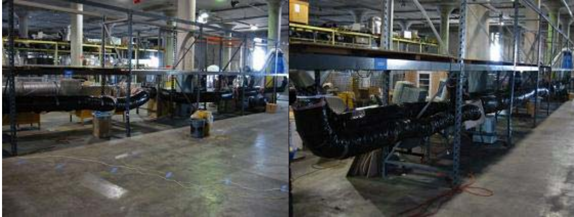
Figure 10. Full Scale multi-branch duct system in LBNL Laboratory
