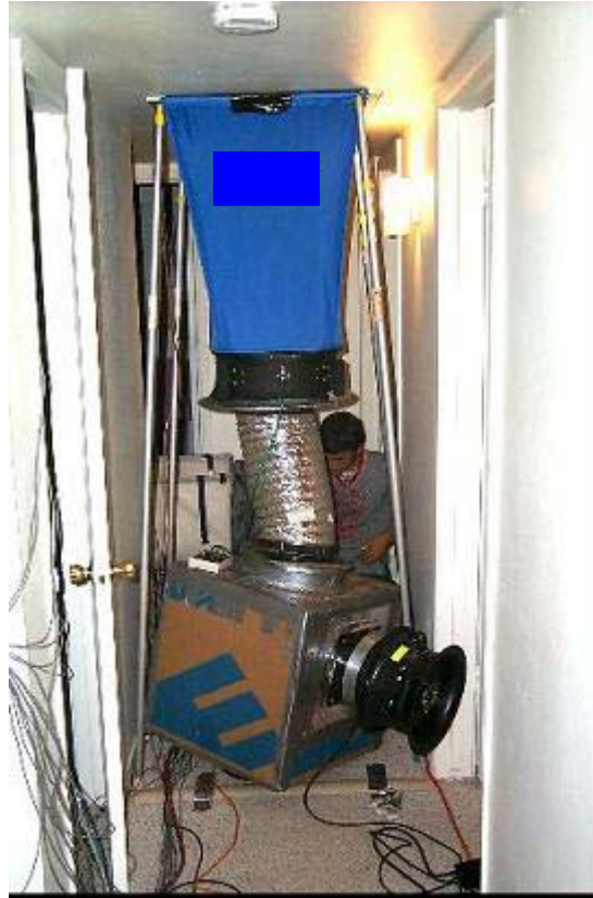
Figure 24. Multiple fan-flowmeter return powered flow hood
