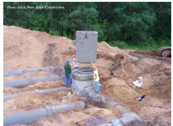
Lowering the air intake tube into place. This piece will remain above-ground.
