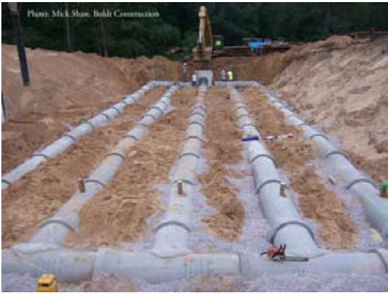
Completed earth tube array
