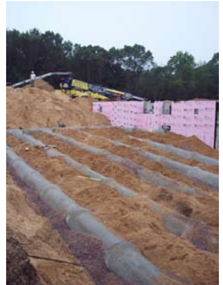
The tubes connect to mechanical ventilation systems in the main building basement
