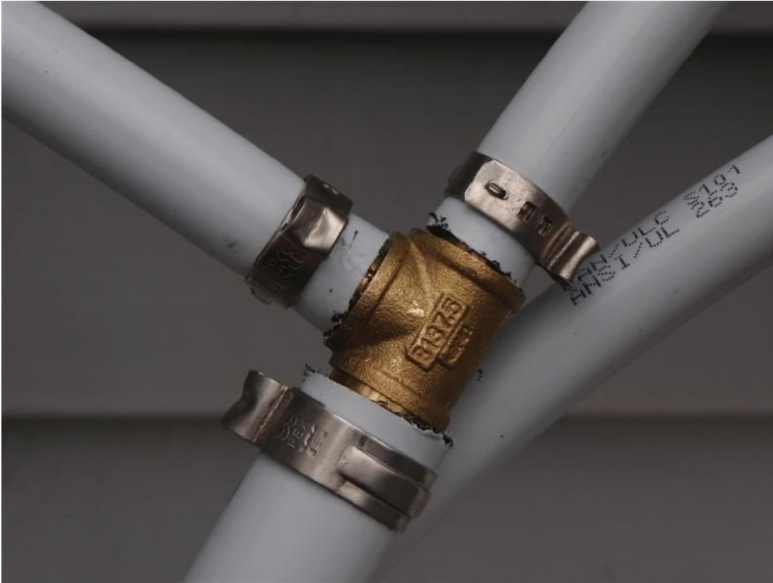
\frac{3}{4} " feed line splitting into two \frac{1}{2} " lines, one for each collector half
